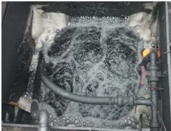
Top view into reactor of test plant
